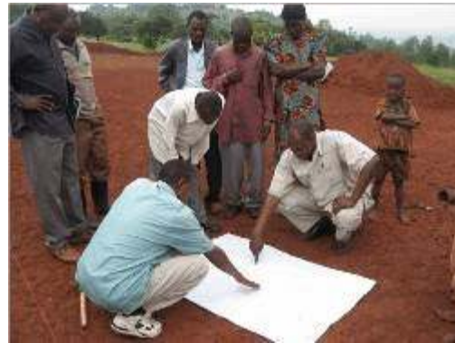
Upper left: Discussion leader; at right: stacking stones for foundation Below: Showing the District Mayor the foundation lines.
