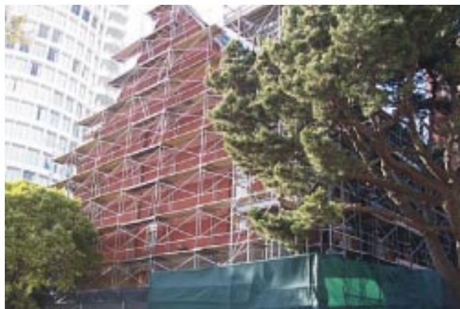
The retrofitting of St Mark's in San Francisco. The congregation is holding all services in the Urban Life Cener buidling, next door to the church building. It will be some months before the job is complete.
